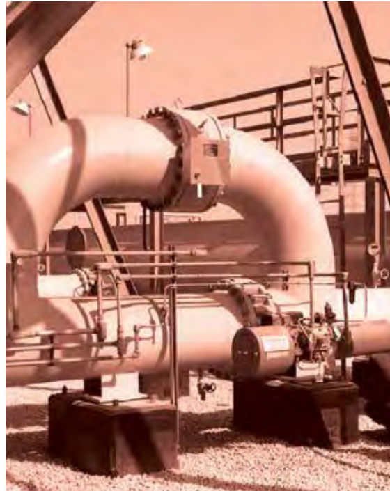
Buckling Pin Relief Valve installed as inline bypass to control valve on a gas flare system
